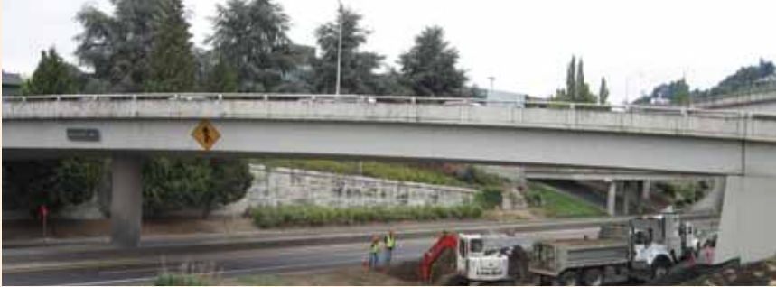
Condition assessment of buried critical pipe at Interstate 405 and SW Taylor and Salmon streets
