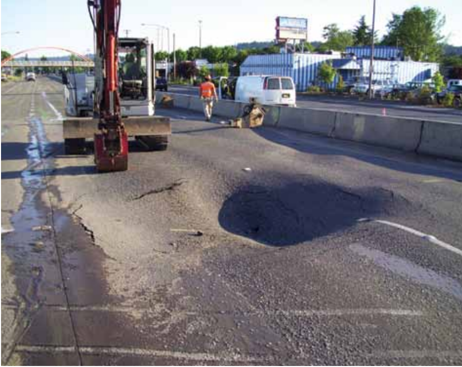
Left: A sinkhole at SE McLoughlin Street in Portland, Oregon.
