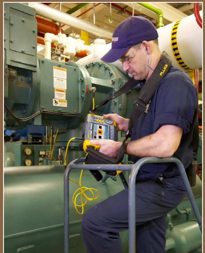
Figure 2: At Alpenrose Dairy, regular vibration analysis provides data for trend analysis used in proactive maintenance
