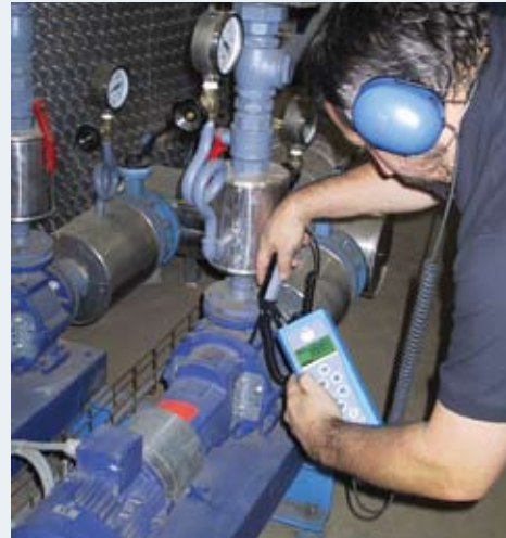
Figure 4 - Monitoring feed water pump
